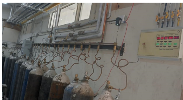
Figure 3: Oxygen cylinder bank with digital gas alarm system
